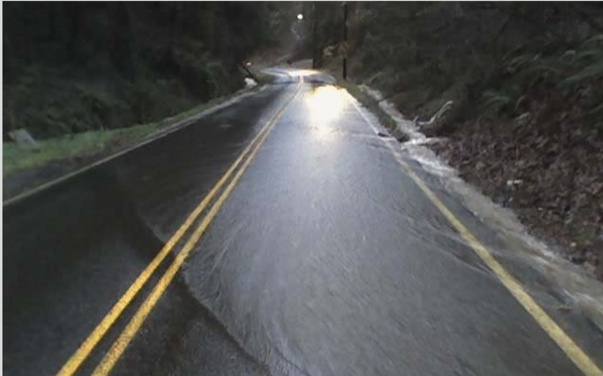
Figure 15. Photos of SE Barbara Welch Blvd During a Heavy Rainstorm, Dec. 2007
