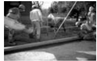
Projects such as this sidewalk on SW Capitol Highway have been constructed with capital funding directed through the Pedestrian Transportation Program.
