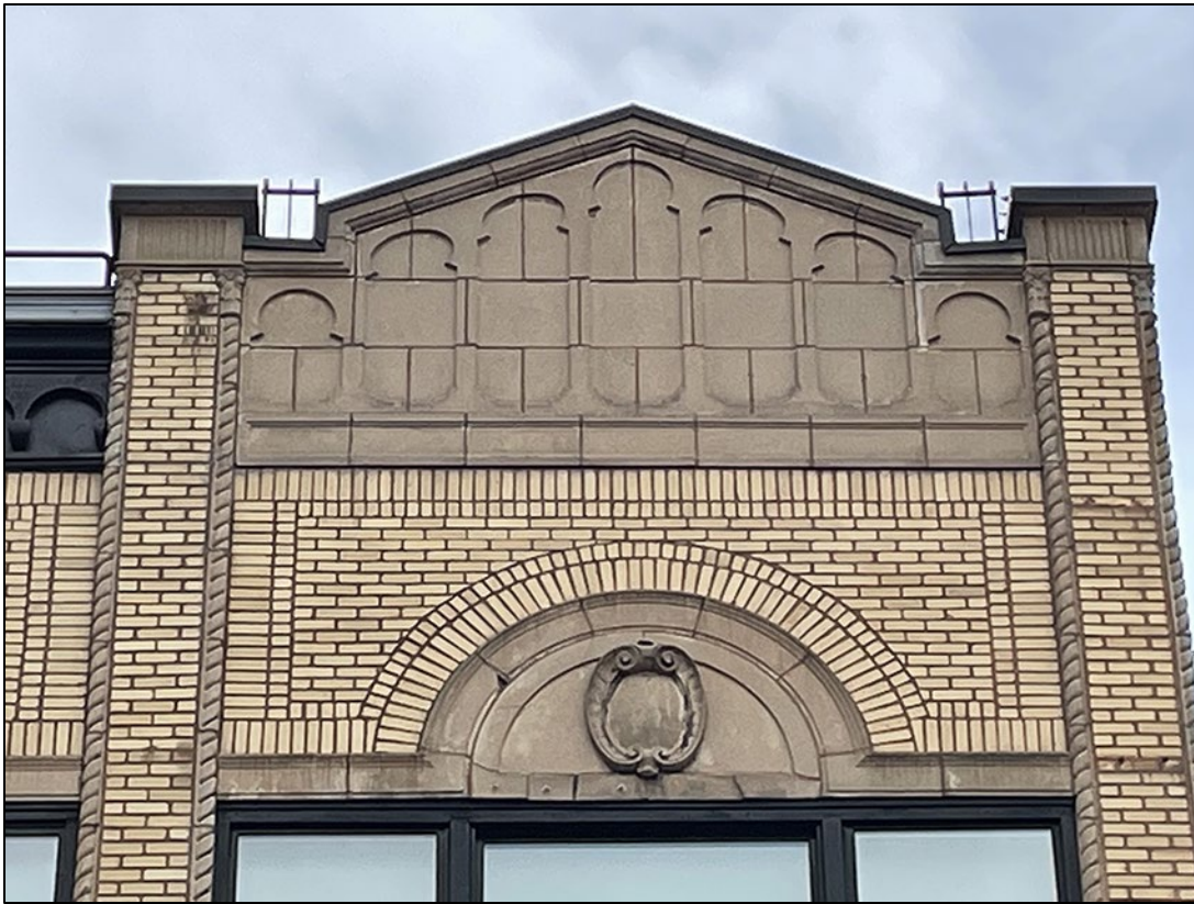
Photo 5 of 12: OR_MultnomahCounty_AlderwayBuilding_0005 Typical corner bay cast stone parapet, south elevation, camera facing north.
