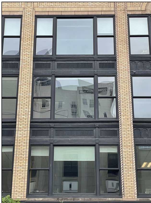
Photo 6 of 12: OR_MultnomahCounty_AlderwayBuilding_0006 Typical Chicago Style window with decorative metal spandrel panel, south elevation, camera facing north.
