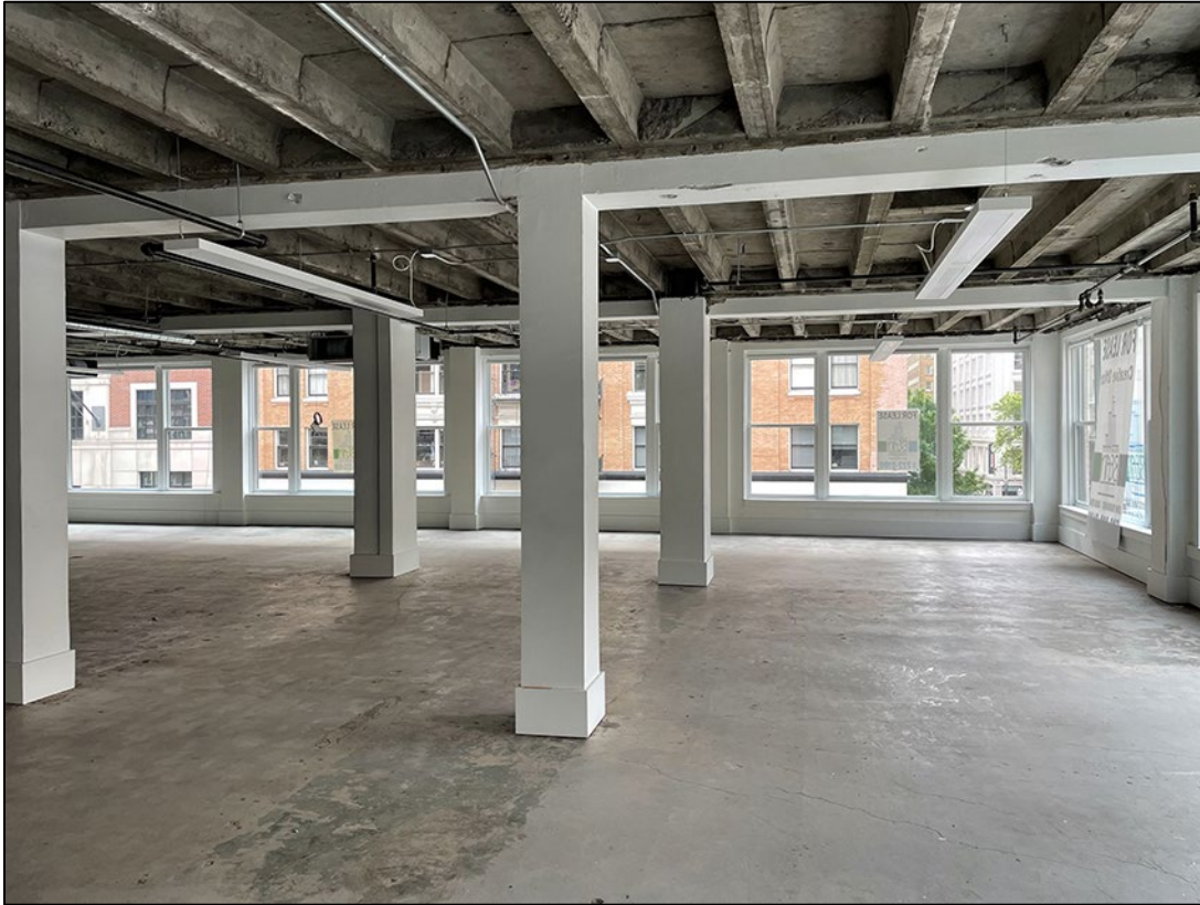
Photo 11 of 12: OR_MultnomahCounty_AlderwayBuilding_0011 Third floor tenant space (vacant at time of photo), camera facing east.
