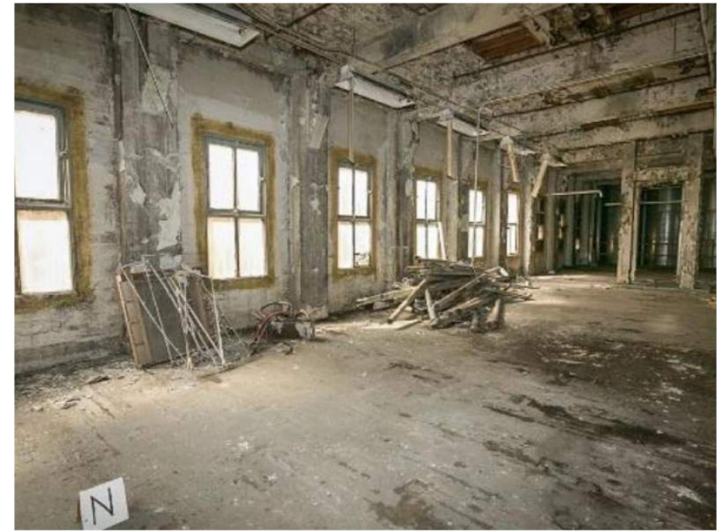
FLOUR MILL INTERIOR CONDITION
