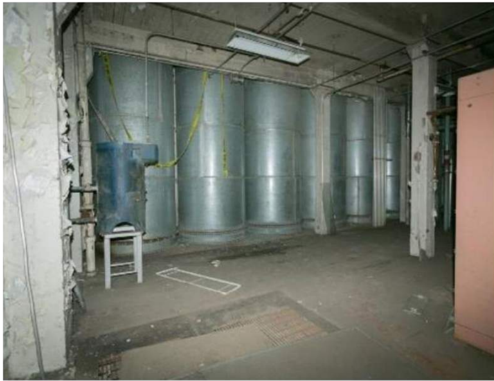
FLOUR MILL INTERIOR CONDITION
