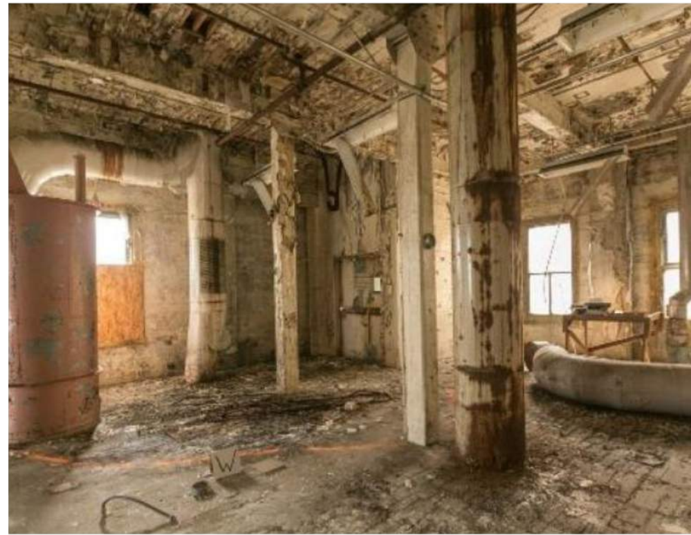
FLOUR MILL INTERIOR CONDITION
