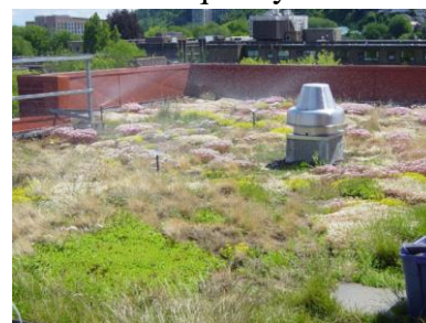
Figure HA-14: Sprinklers on Hamilton Ecoroof
