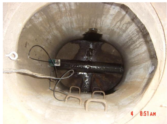
Figure 3-3: Flow sensors installed in sewer
