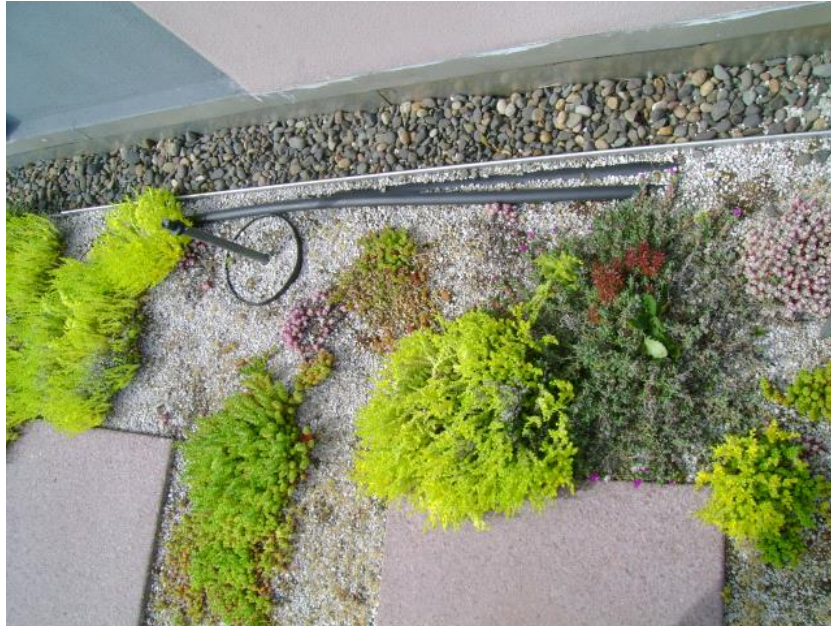
Figure PB-10: Exposed HDPE irrigation lines near the penthouse wall
