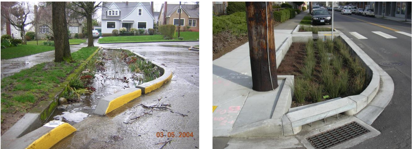
Figure 5-3: Green Street Curb Extensions at NE 35 th & Siskiyou (left) and SE Belmont & 42 nd (right)
