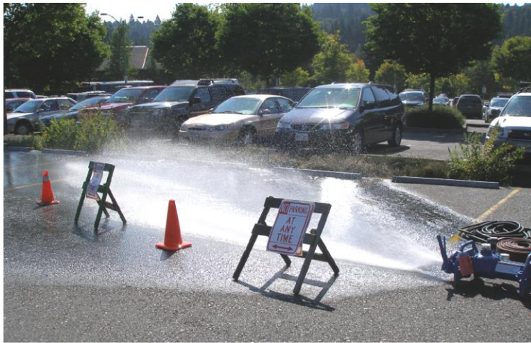
Figure OZ-6 – flow test of Row #7 (flow rate approximately 56 gpm)
