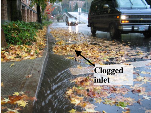
Figure SW-7: Flow bypassing a clogged inlet just above the facility
