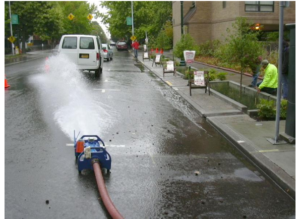
Figure 3-4: Flow test at SW 12th & Montgomery Green Street
