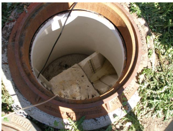
Figure RC-2: Monitoring manhole
