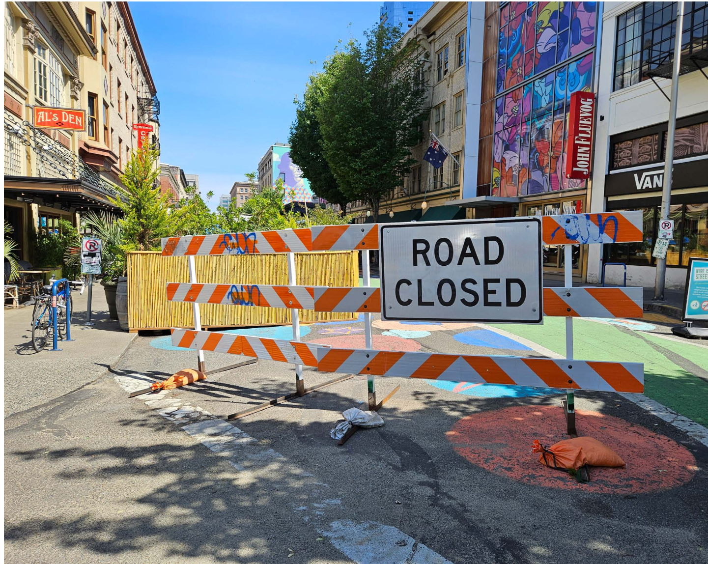
Pride Plaza Standard Traffic Signage for Road Closures
