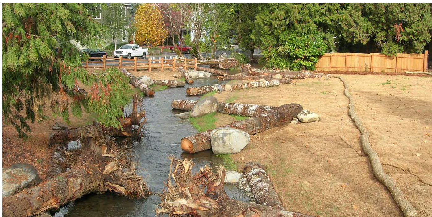
Restoration of Crystal Springs Creek between SE Tenino Street and SE Umatilla Street. Two culverts were replaced to provide fish passage and large wood and boulders were added to the channel to provide habitat.
