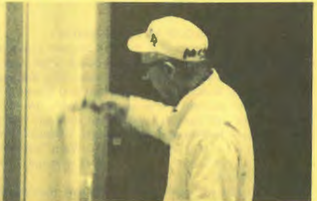
Roy Blomberg, maintenance paint crew, adds the finishing touches to one of the new recreation office walls.
