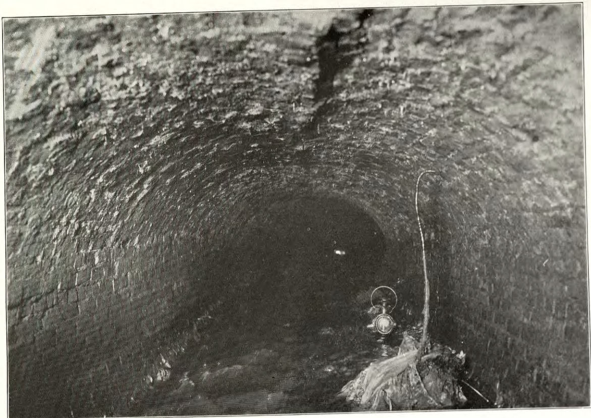
View of Tanner Creek Sewer at 12th and Everett Streets, showing dangerous crack in arch. (Taken October 17, 1913.)
