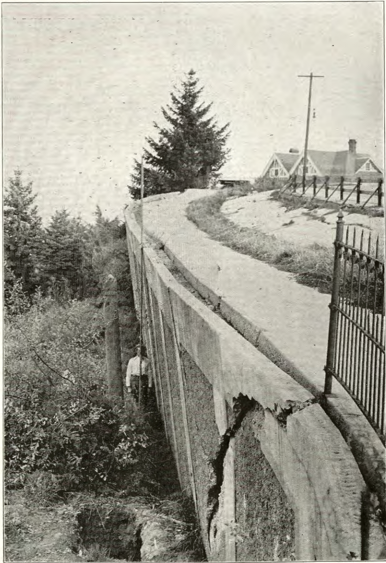
Illustration showing failure of original Vista Avenue Retaining Wall. (Taken September 23, 1913.)
