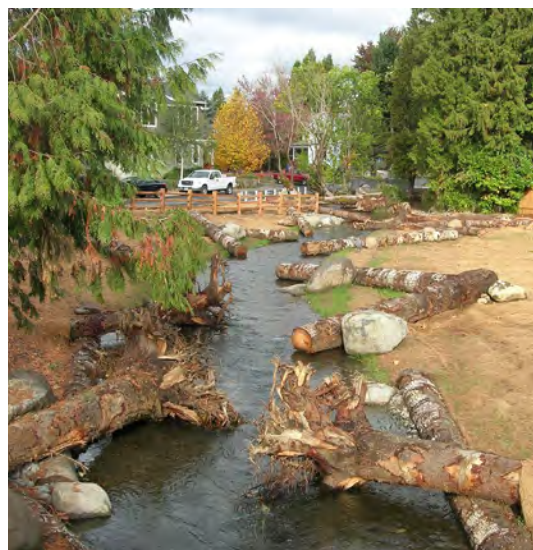
Restoration of Crystal Springs Creek between SE Tenino Street and SE Umatilla Street. Two culverts were replaced to provide fish passage and large wood and boulders were added to the channel to provide habitat.
