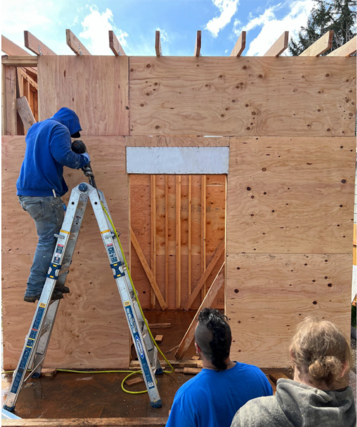
A Cascadia Clusters Trainee “skinning” Unit #2 at the 12 & 12 Village on Glisan we are currently building in partnership with City Team and the Arabic Life Church (16001 NE Glisan). All materials were donated by Woodland Wood Connections.
