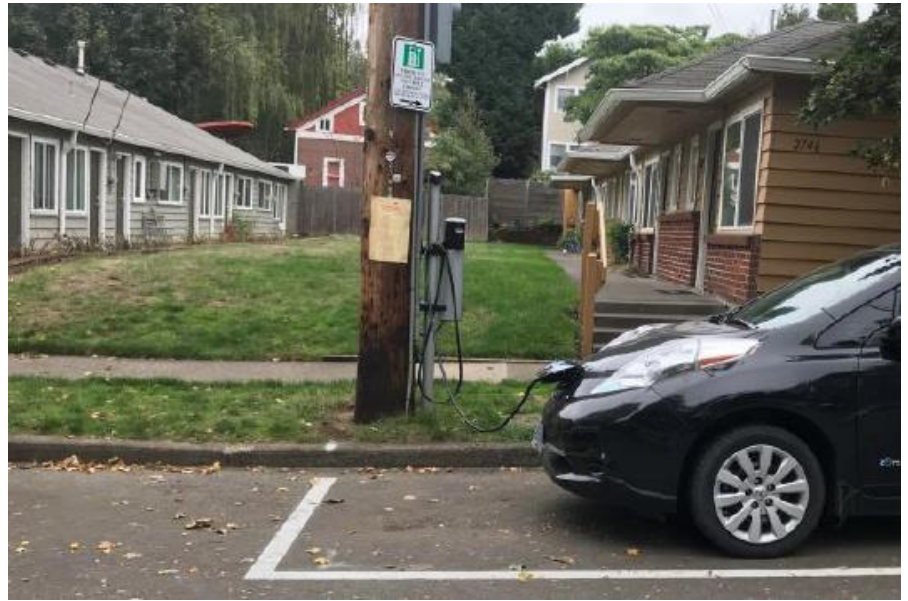
Pole-mounted L2 charger in SE PDX
