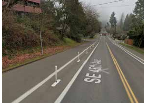
SE 45th Ave sidewalk gap
