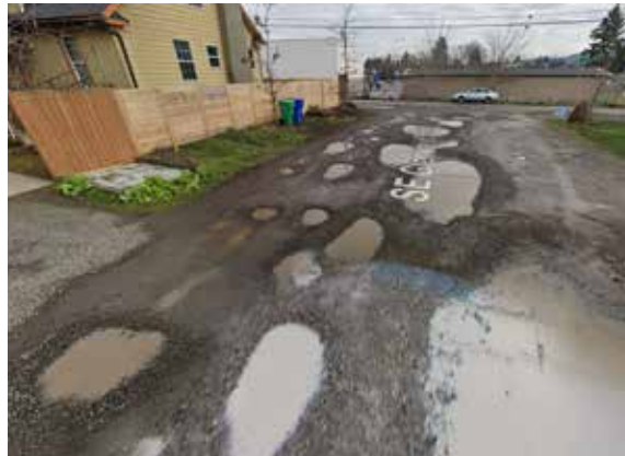
Water-filled potholes on SE Glenwood St
