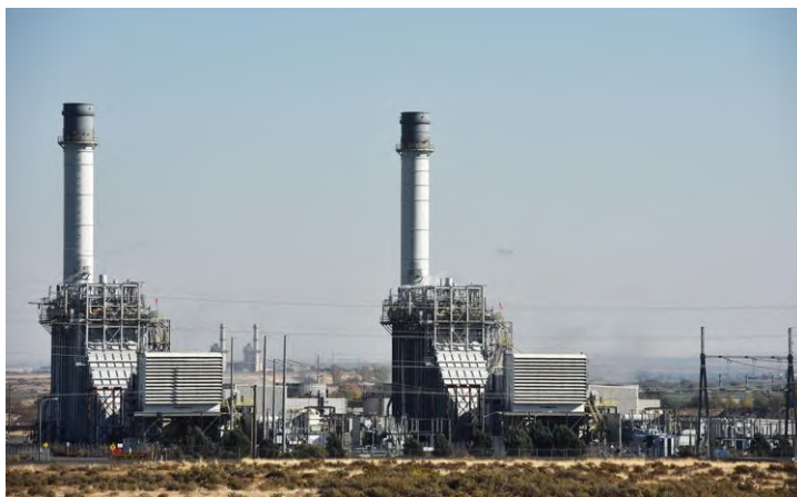
The Hermiston Generating Plant provides power for nearly 500,000 households in the Pacific NW, courtesy of Perennial Power.
