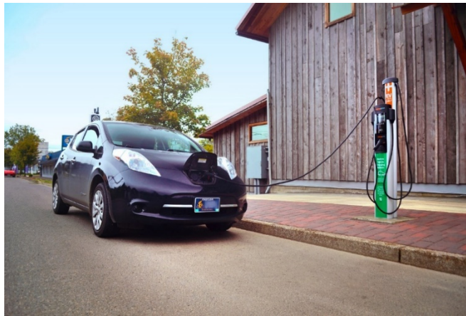
Figure 42. An Electric Vehicle Charges at a Level 2 Charging Station Funded Through the Grant in Philomath, Oregon
