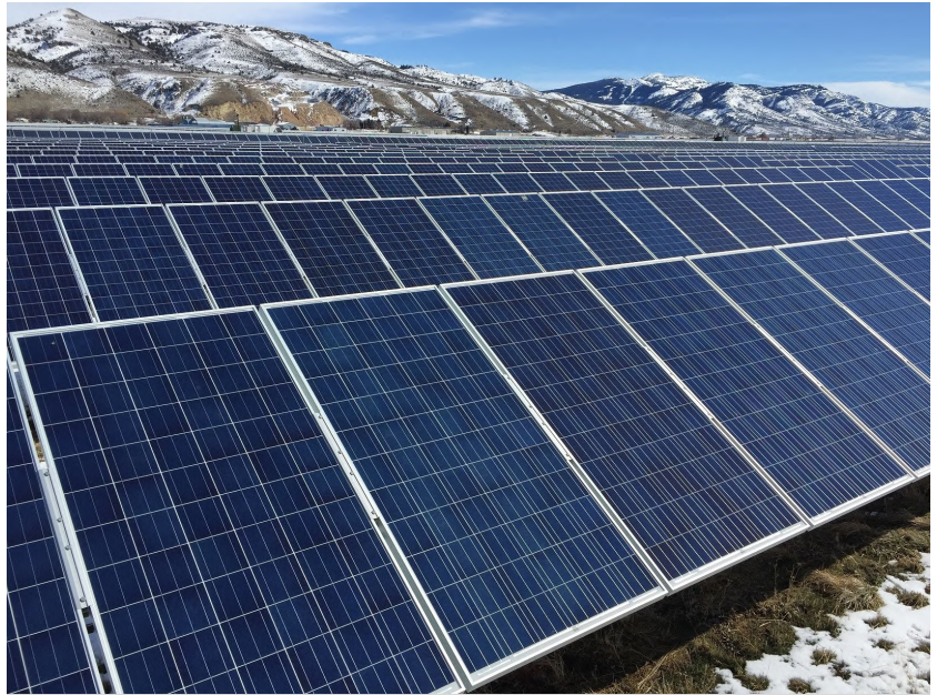
PacifiCorp's 2-megawatt Black Cap Solar facility in Lakeview, OR.
