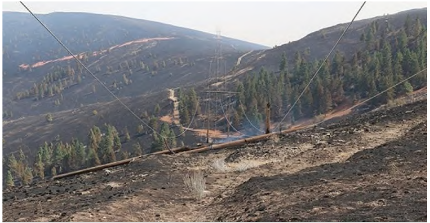
Wildfire knocked out BPA's Hot Springs-Rattlesnake 230-kV line in Montana in August 2015 46
