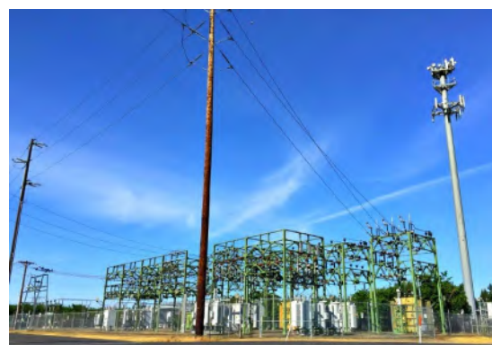
Substation in Canby, Oregon.
