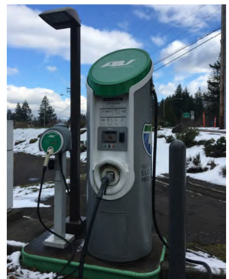
West Coast Electric Highway Charger in Cascade Locks.
