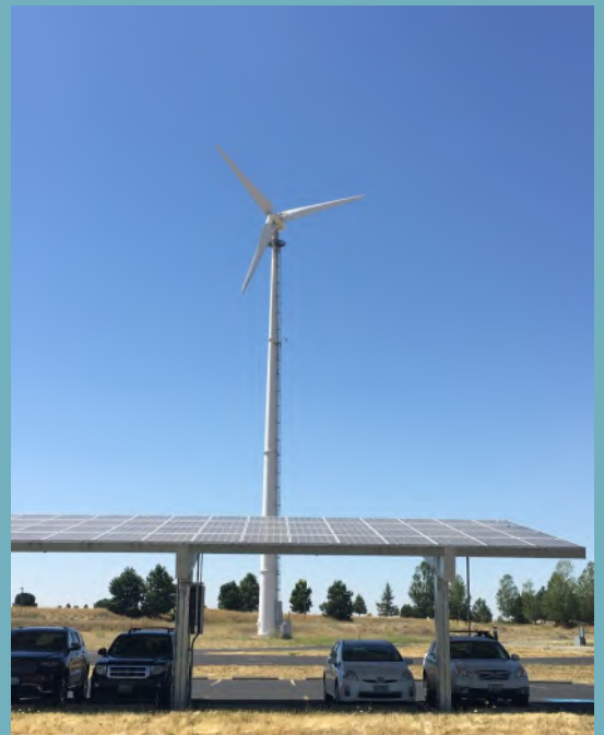
Wind turbine and solar array at the Tamástslikt Cultural Institute
