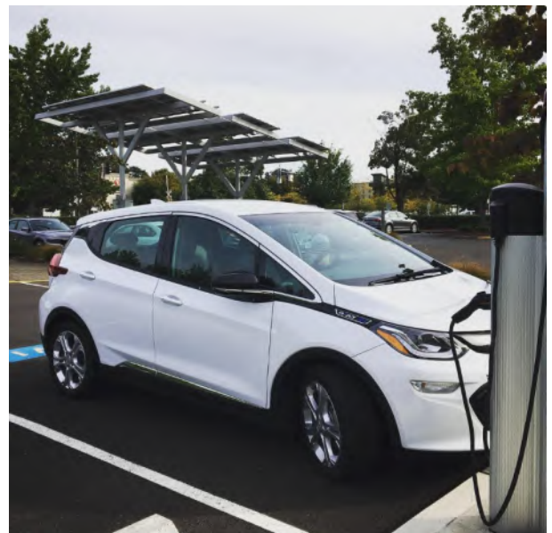
The State of Oregon’s “550” Building has electric vehicle chargers and a 8,300 watt solar array.
