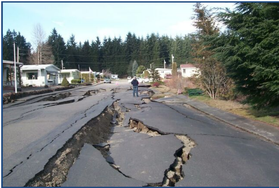
Figure 1-4. Damaged road due to liquefaction-induced lateral spreading, 2001 Nisqually, Washington earthquake. Photographic credit: DOGAMI Archives.
