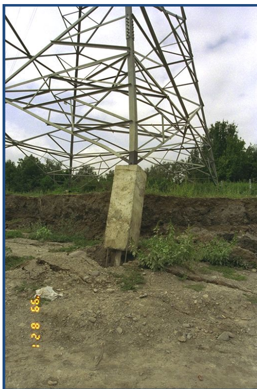
Figure 1-3. Example of ground failure underneath a transmission tower, 1999 İzmit earthquake (Turkey). Photographic credit: University of California, Irvine Consortium of University for Research in Earthquake Engineering Archives.
