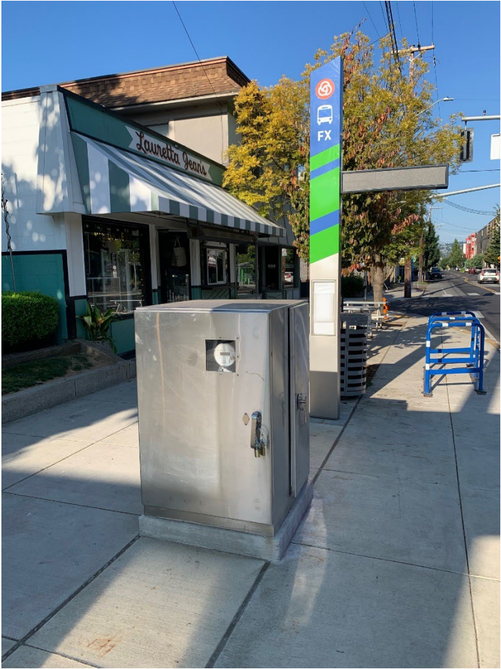
Platform Comms/Power Cabinet
