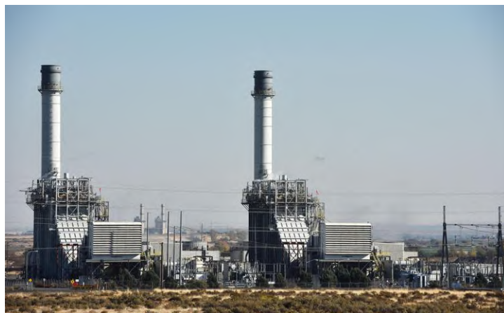
The Hermiston Generating Plant provides power for nearly 500,000 households in the Pacific NW, courtesy of Perennial Power.
