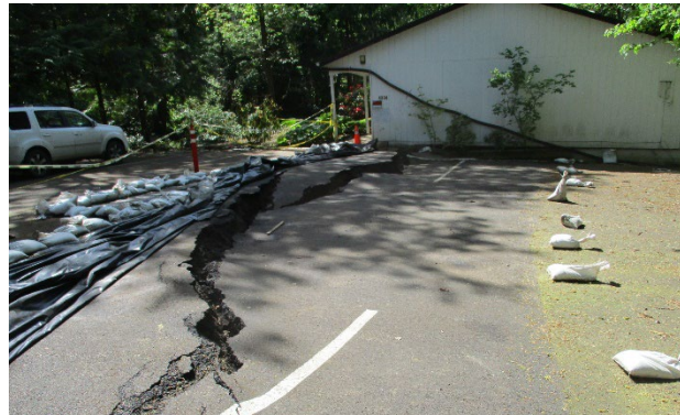
Example of an active deep landslide
