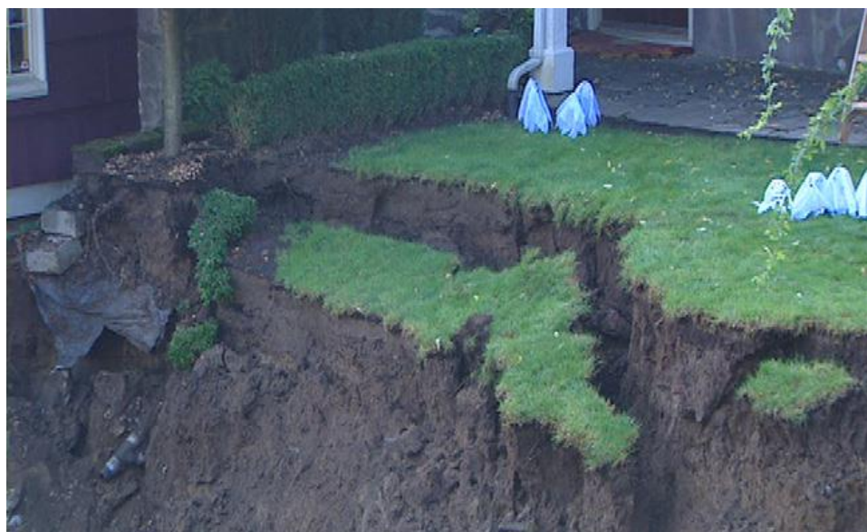
Image: Landslide in Southwest Portland (2008)
