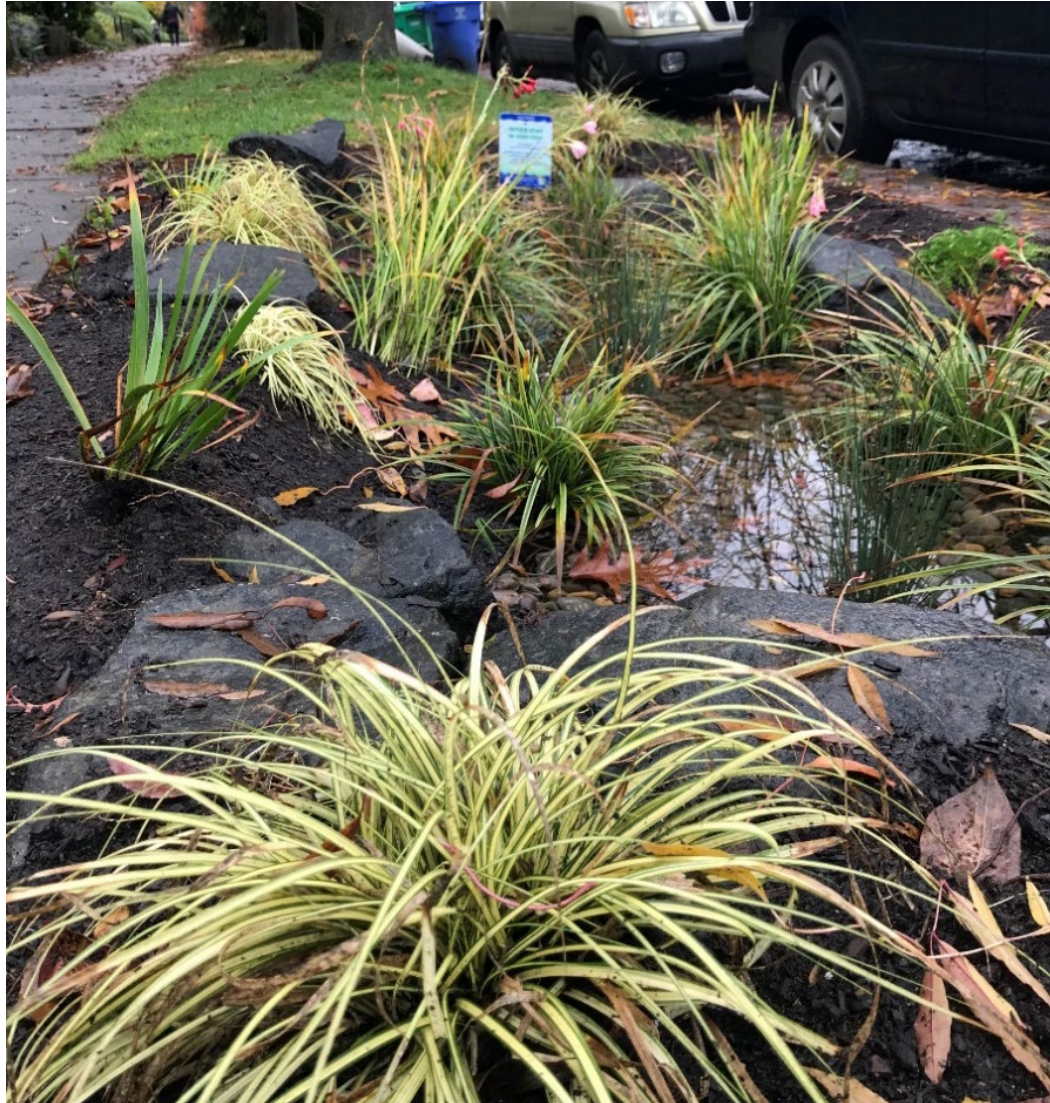
Figure 18 Example retrofit #3, SE Richmond ROW Rain Garden in action
