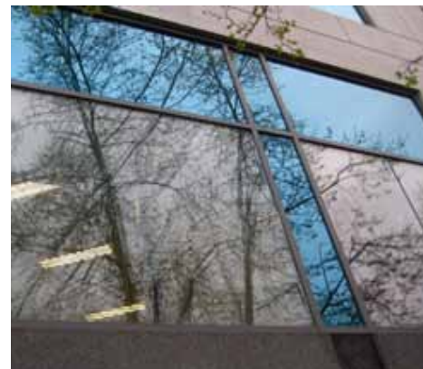
Tinted windows at the State Building readily reflect vegetation. More testing on colors and density is needed. Photo: Mary Coolidge
