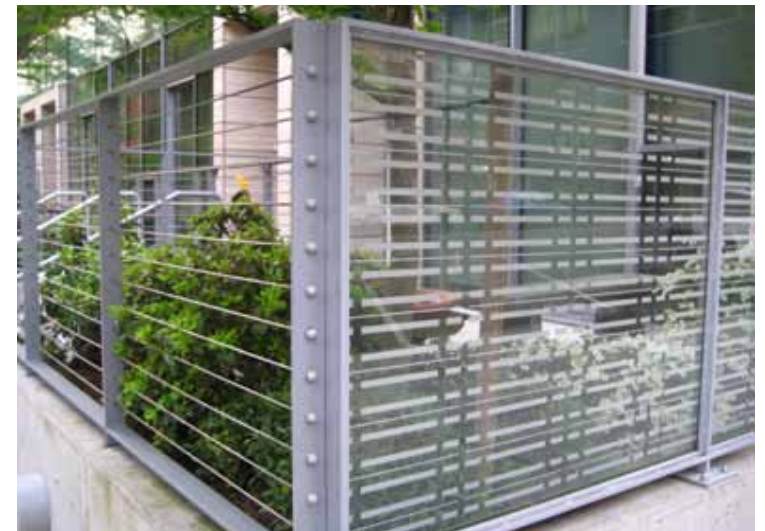
Visual markers on the balcony glass at the Eliot Tower provide some privacy and decrease strike hazards. Photo: Mary Coolidge
