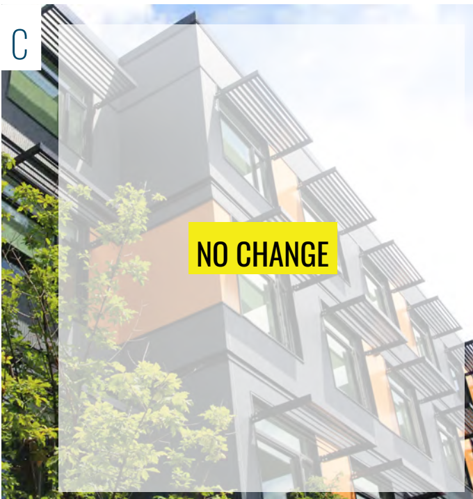
Providing sunshades along southern and western sides of buildings. Sunshades can reduce temperatures where sun exposure is direct, and they create deep shadows to reduce bird strikes. MLK, NE Martin Luther King, Jr. Blvd and NE Monroe
