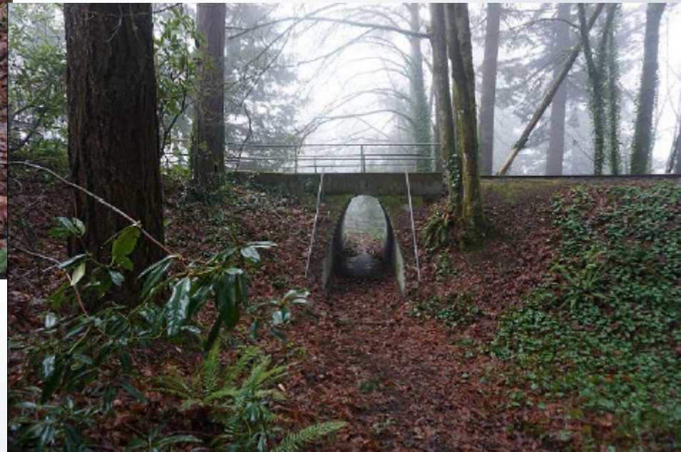
Viaduct over Path to Platform at Washington Park Station looking East Today
