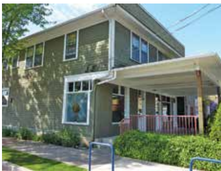
Wood frame structure with its single story front load bearing wall replaced by concrete block, this renovation may be a liability.
