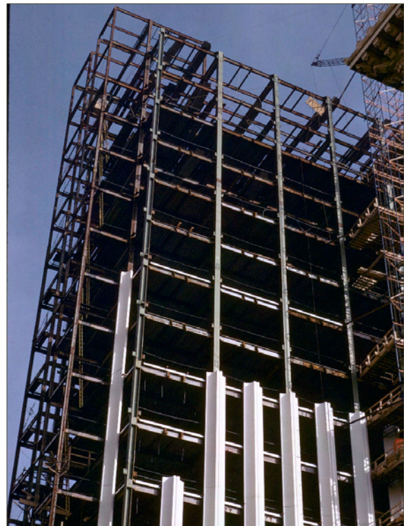
The Bank of America tower, with its curtain wall structure is shown in construction (1968) at 1001 SW 5th Ave.
