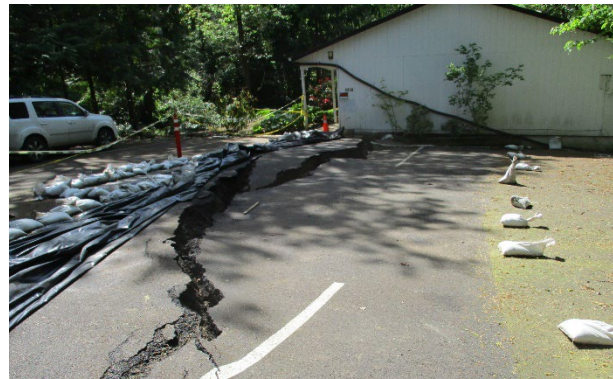
Example of an active deep landslide
