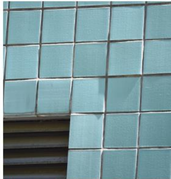
Out of plane tiles potentially delaminated from wall
