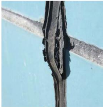
Failed sealant at tile system control joint
