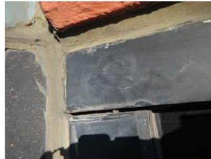
Complex material transition joints dependent on sealant
