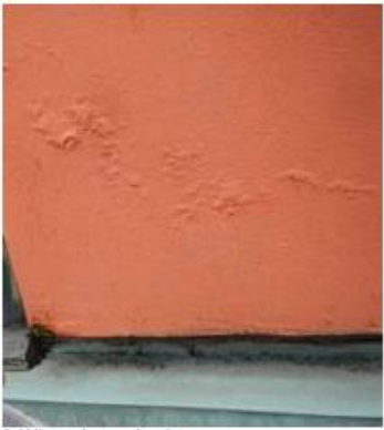
Bubbling at elastomeric paint
