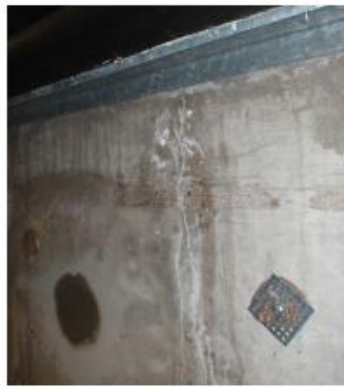
Water staining on interior side of concrete wall
