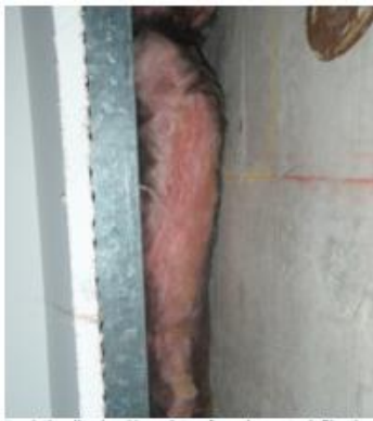
Insulation discolored by moisture from air or water infiltration
