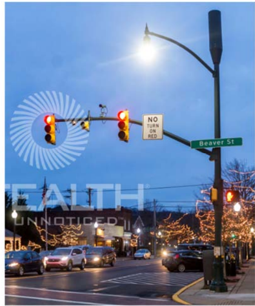
A positive small cell example on a traffic signal pole with stealth and camouflage features.
