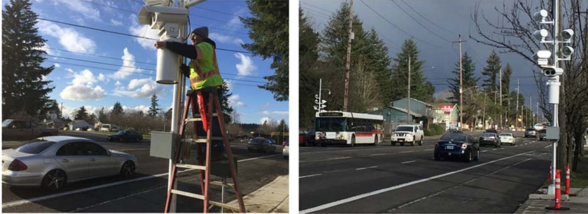
Images of fixed speed safety cameras being installed and deployed to on Portland roadways. (Images from PBOT's New Release "Speed Safety Cameras start issuing warnings today on two East Portland high crash corridors").
