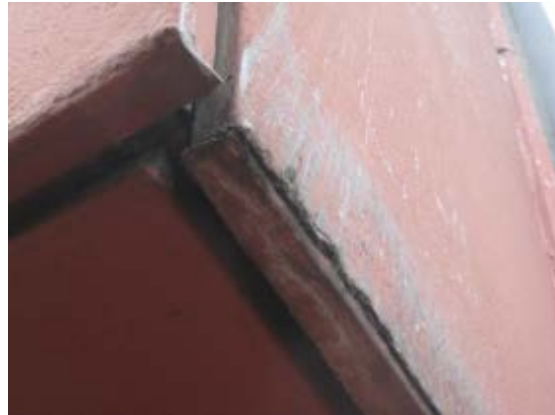
88. Stucco Omitted Sealant Joints
