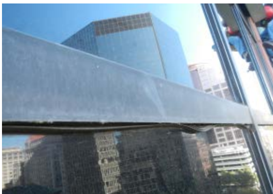
41. Curtainwall Failed Glazing Gaskets
