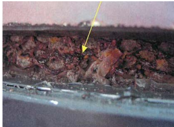
67. Corroded Metal Lath at Ribbon Window head
