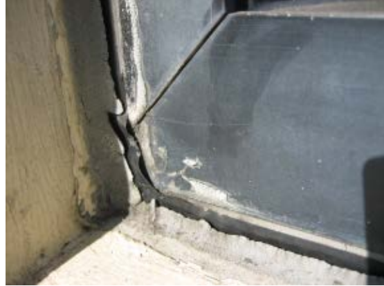
27. 'Punched' Window Joinery Failure
