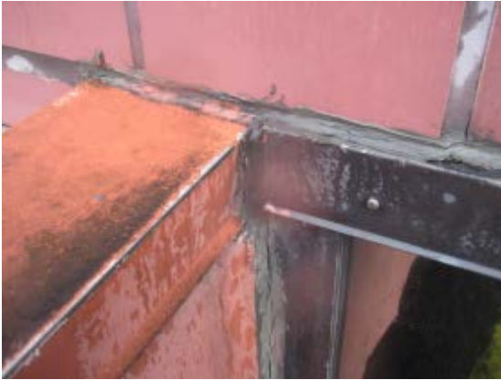
44. Curtainwall Failed Perimeter Sealant
