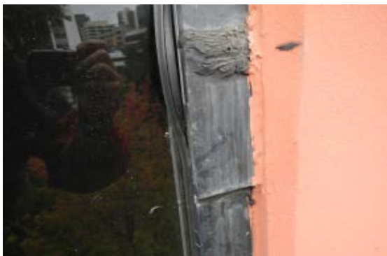
49. Curtainwall Failed Expansion Joints
