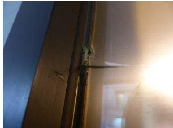
34. Storefront Cracked Glazing
