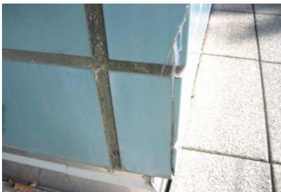
66. Ceramic Tile, Cracked, Sealant Failure
