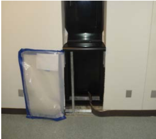
6. Test Site 4-10 Wall opened up for observation
