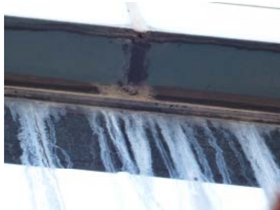
28. 'Punched' Window Finish Damage
