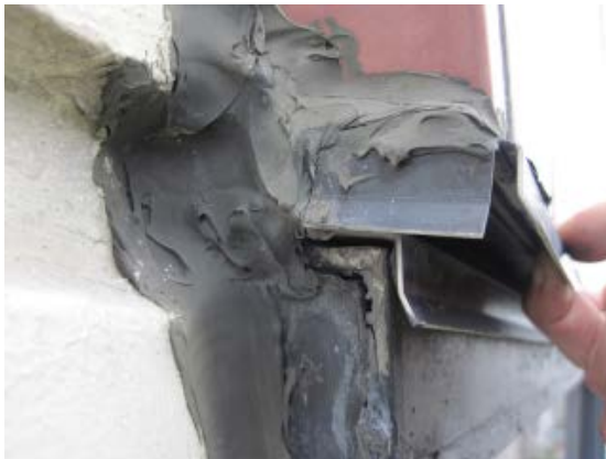
61. Ribbon Windows Failed Flashing Detail
