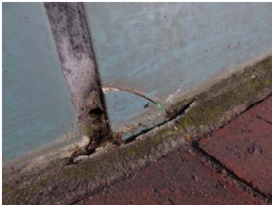
65. Ceramic Tile, Cracked, Sealant Failure
