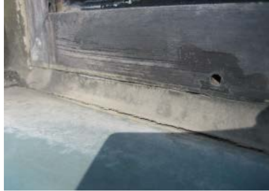
42. Curtainwall Failed Perimeter Sealant
