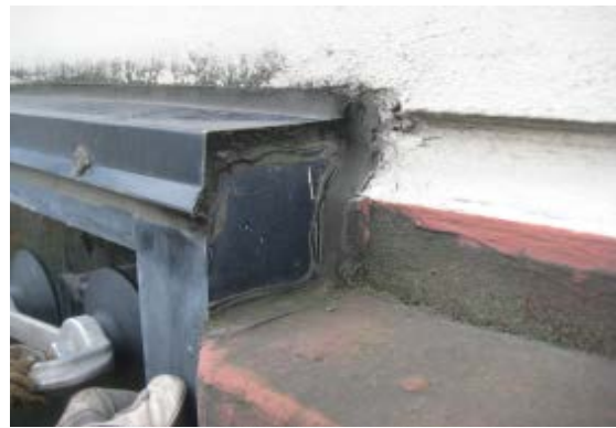
45. Curtainwall Inadequate Flashing Detailing
