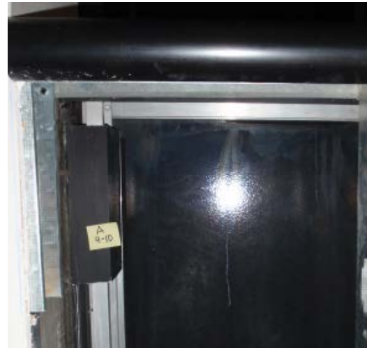
99. 9.10 Moisture Stains on Spandrel Panel
