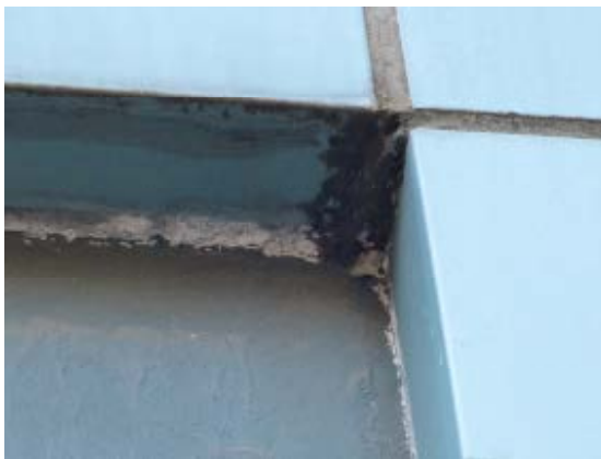
69. Ceramic Tile, Efflorescence
