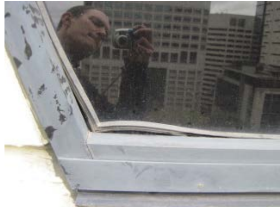
24. 'Punched' Window Gasket Failure
