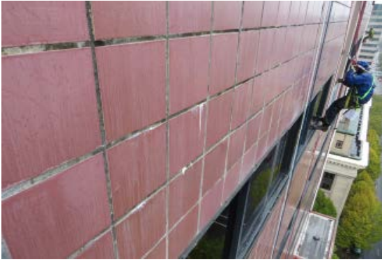
2. Exterior Inspection of Red Ceramic Tile and Ribbon Windows by boson's Chair.
