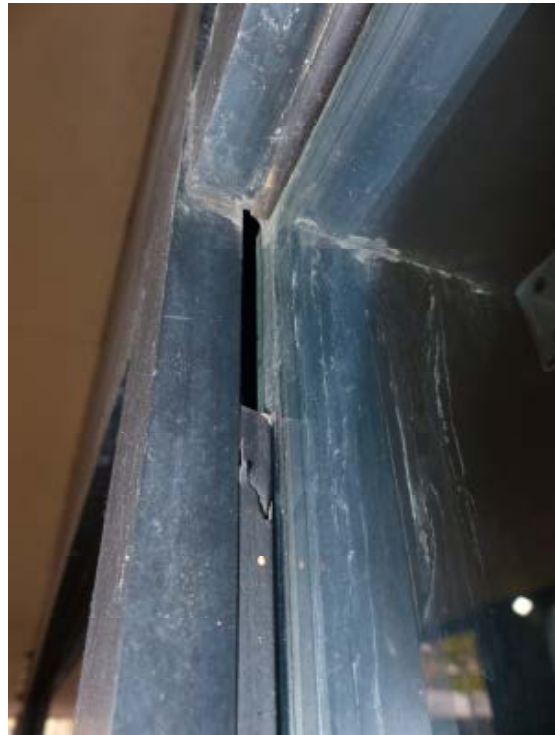
32. Storefront Failed Glazing Gasket
