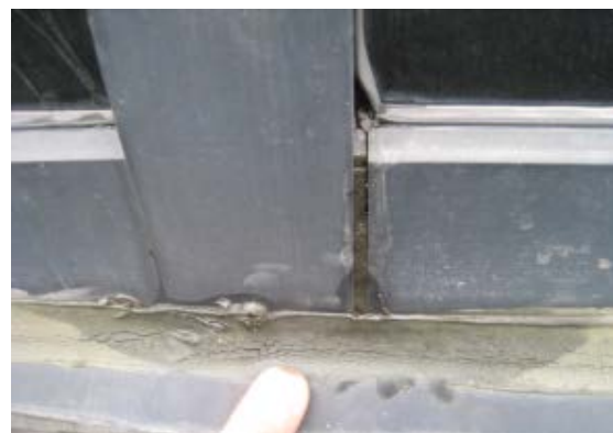
50. Curtainwall Deteriorated Joinery Seals
