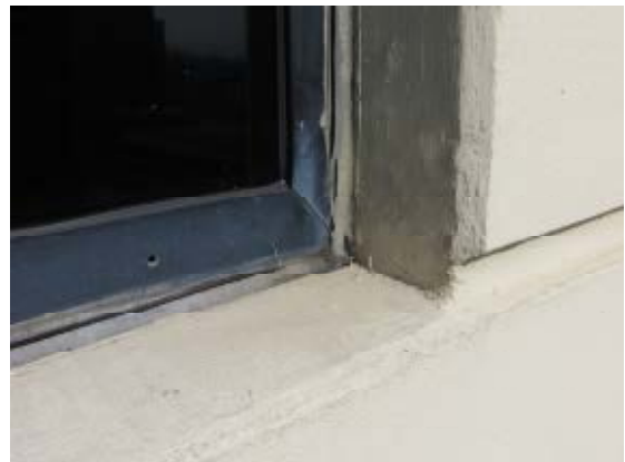
25. 'Punched' Window Sealant Failure
