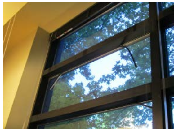
5. Interior Assessment Storefront SSF6 Close-up (note: failed glass gaskets)
