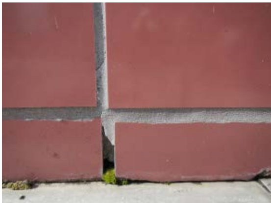
74. Ceramic Tile Ineffective Re-pointing
