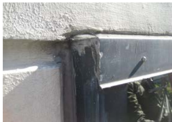
46. Curtainwall Inadequate Flashing Detailing
