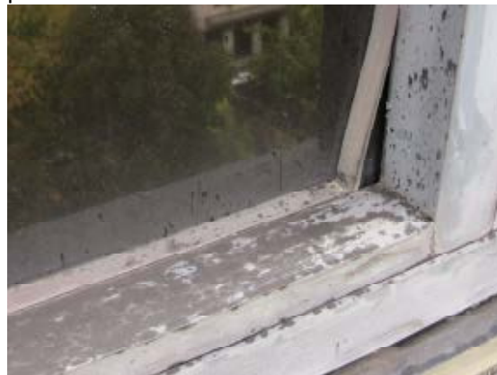
53. Ribbon Windows Failed Gaskets
