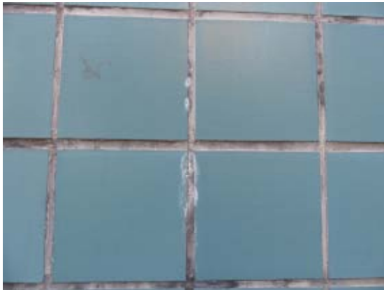
68. Ceramic Tile, Efflorescence
