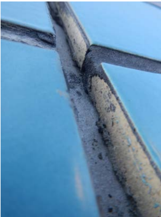
77. Ceramic Tile Sealant Failure
