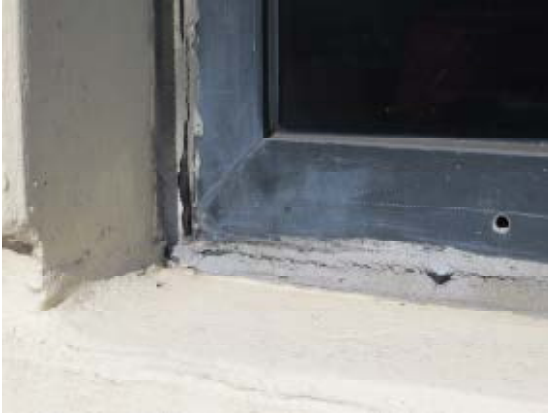
29. 'Punched' Window Finish Damage
