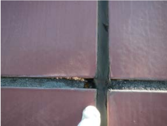
76. Ceramic Tile Sealant Failure
