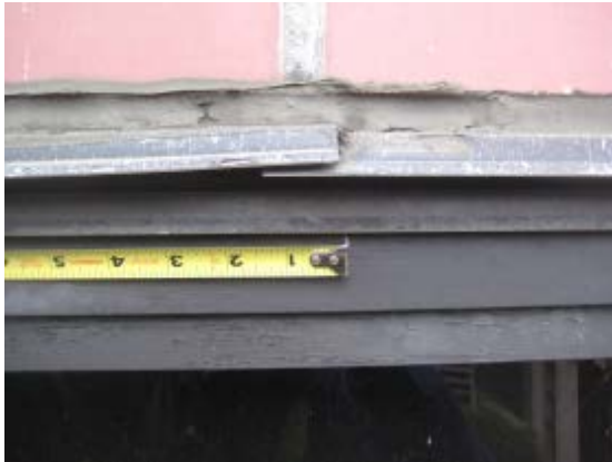
60. Ribbon Windows Failed Flashing Detail
