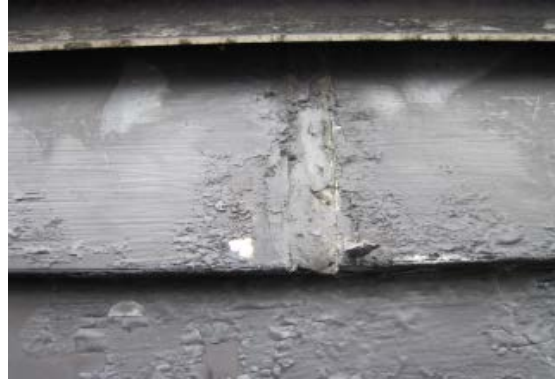
58. Ribbon Windows Deteriorated Finish
