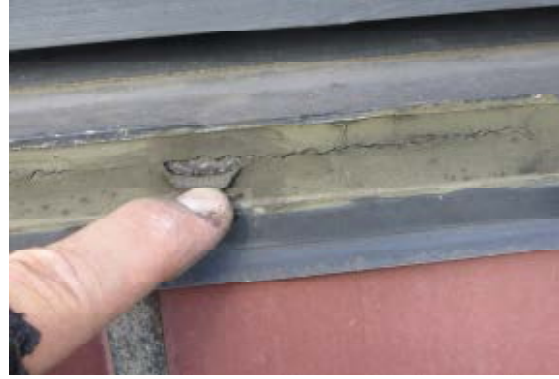
56. Ribbon Windows Failed Perimeter Sealant
