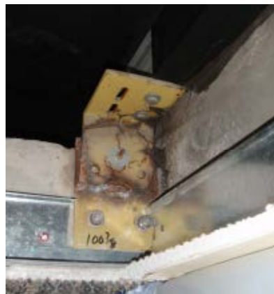
97. 7.10 Water Stains at Connection Plates
