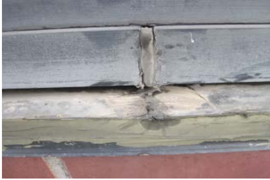
56. Ribbon Windows Failed Expansion Joint Sealant
