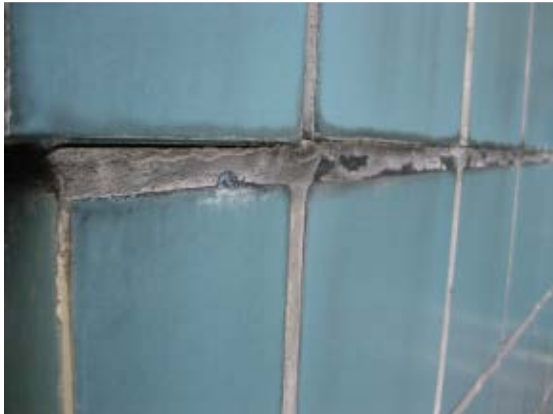
73. Ceramic Tile Ineffective Re-pointing Sealant Failure
