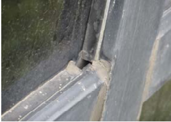
39. Curtainwall Failed Glazing Gaskets
