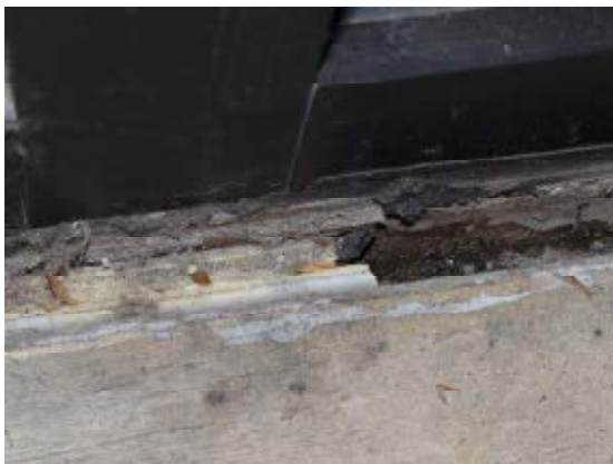
33. Storefront Inadequate Flashing
