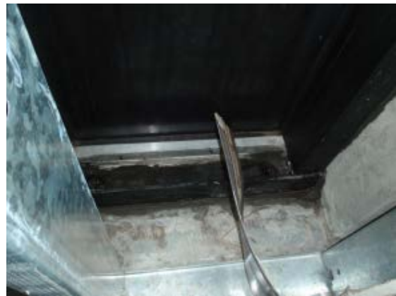
92. 4.10 Sill Track Standing Water
