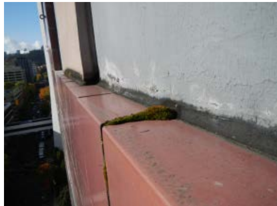
75. Ceramic Tile Exposed Horizontal Joints and Sealant Failure
