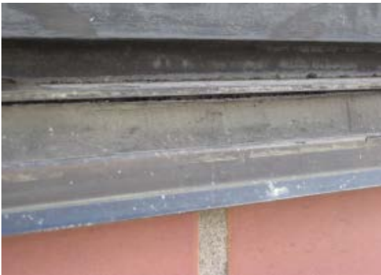
55. Ribbon Windows Failed Perimeter Sealant
