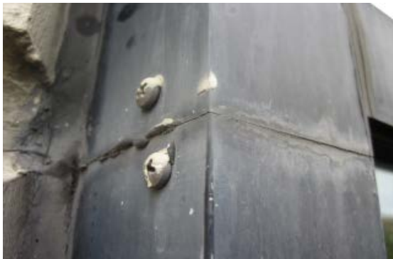
48. Curtainwall Failed Expansion Joints
