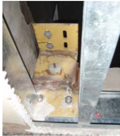
96. 7.10 Water Stains at Connection Plates
