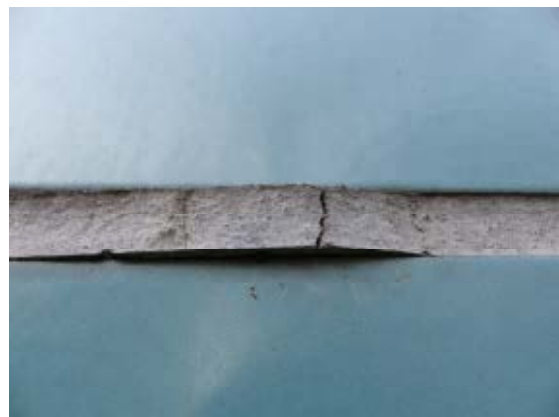
71. Ceramic Tile Deteriorated Mortar Joints
