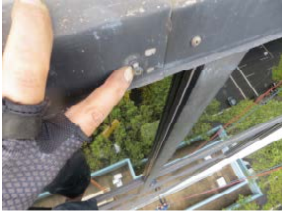
47. Curtainwall Inadequate Flashing Detailing
