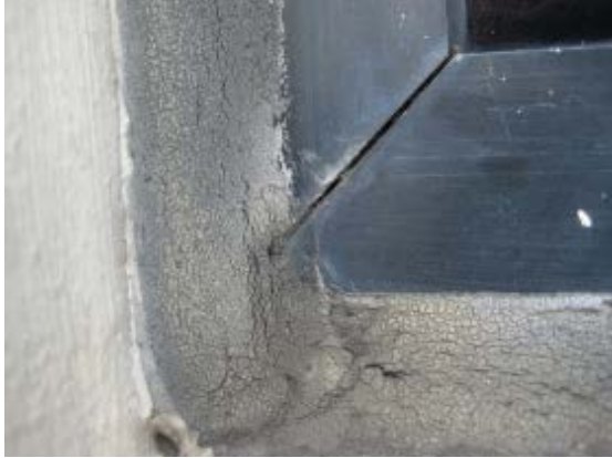
26. 'Punched' Window Sealant Failure
