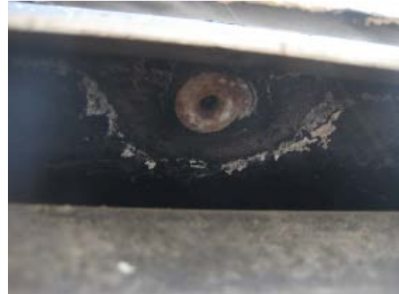
62. Ribbon Windows Corroding Flashing Fasteners
