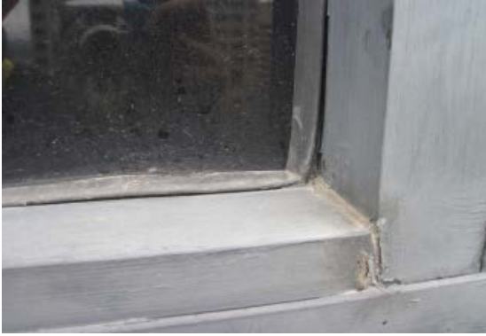
54. Ribbon Windows Failed Gaskets and Finish
