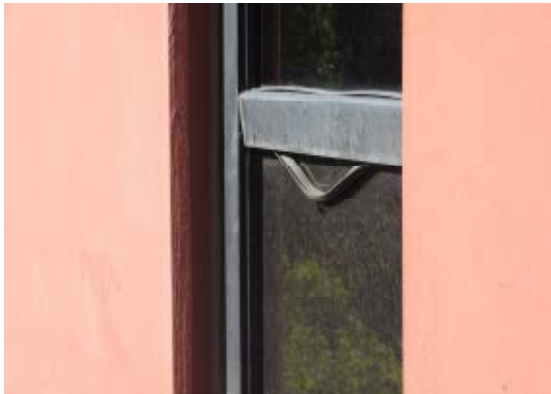
40. Curtainwall Failed Glazing Gaskets
