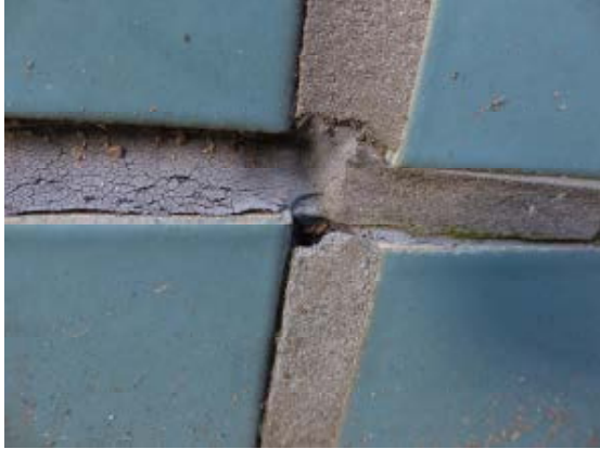
72. Ceramic Tile Ineffective Re-pointing Sealant Failure
