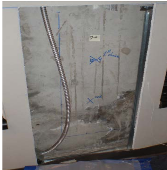
10. Test Site 15-7 opened, Extensive moisture penetration at hairline cracks in concrete wall was noted.
