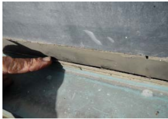
43. Curtainwall Failed Perimeter Sealant
