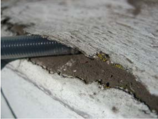
84. Concrete Elastomeric Paint Failure
