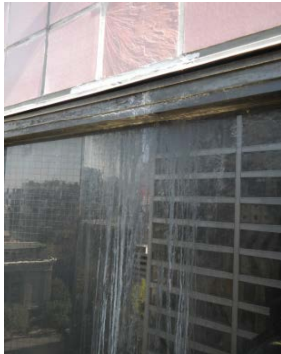
59. Ribbon Windows Corroding Window Frames
