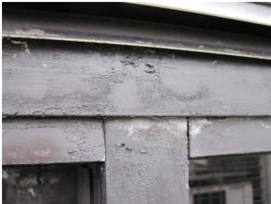
57. Ribbon Windows Deteriorated Finish
