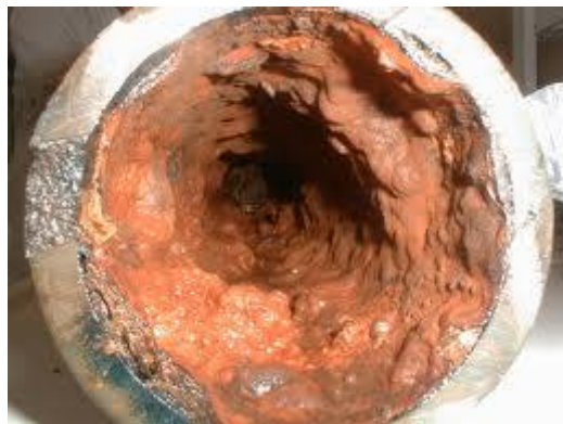
Appearance of biofilm buildup in water distribution pipes due to neglected flushing
