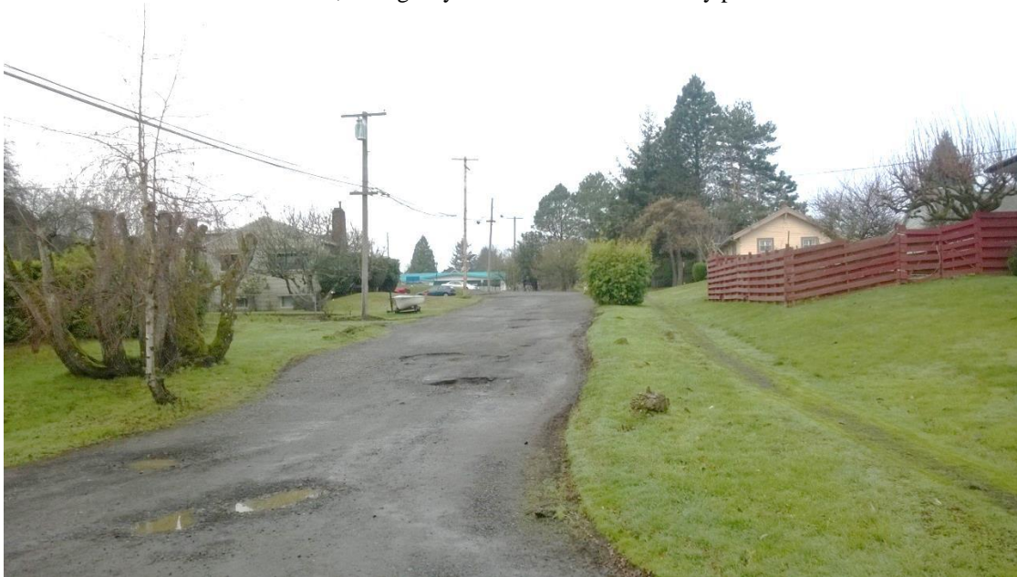
SW Carson Street, east of SW Terwilliger. A severely under-improved and narrow roadway.
