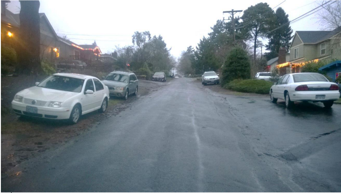
SW 10 th Avenue, between SW Carson and SW Hume Street. A narrow and under-improved roadway. No sidewalks, curbs, or gutters.
