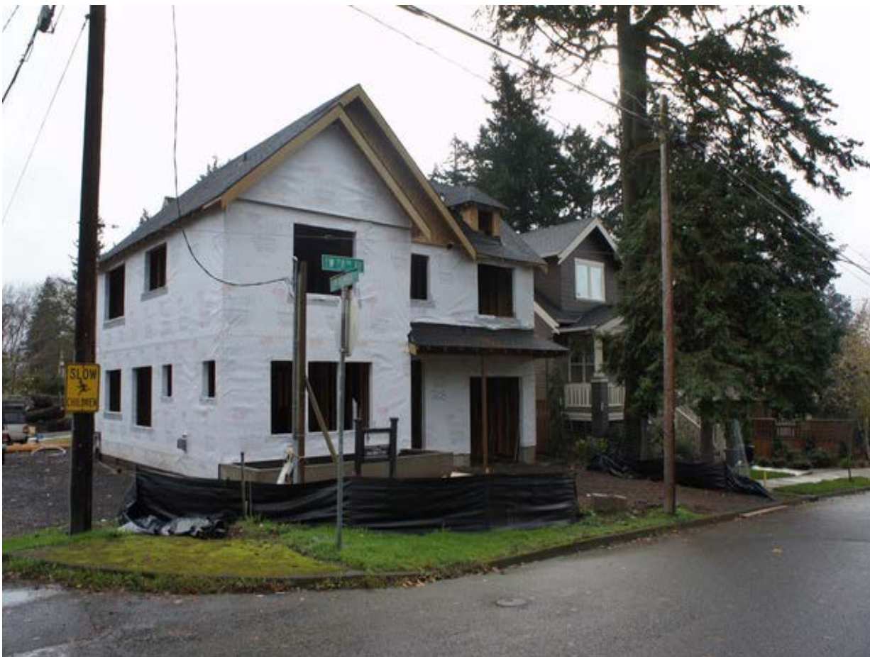
Previous dilapidated home on a corner lot redeveloped as single family home plus duplex.
