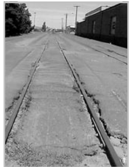
Deteriorating pavement on N. Bradford.
